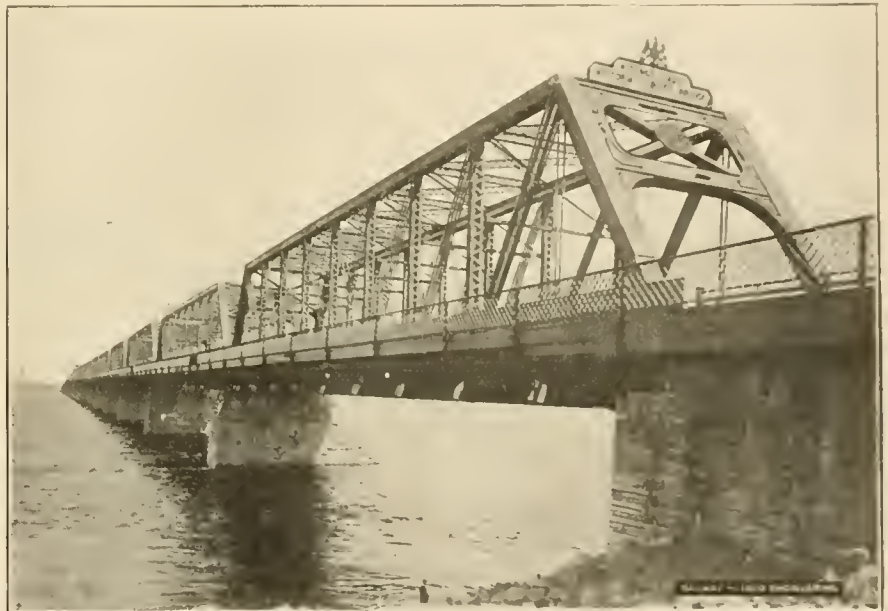
VICTORIA JUBILEE BRIDGE OVER THE ST. LAWRENCE RIVER ON THE GRAND TRUNK SYSTEM AT MONTREAL.
